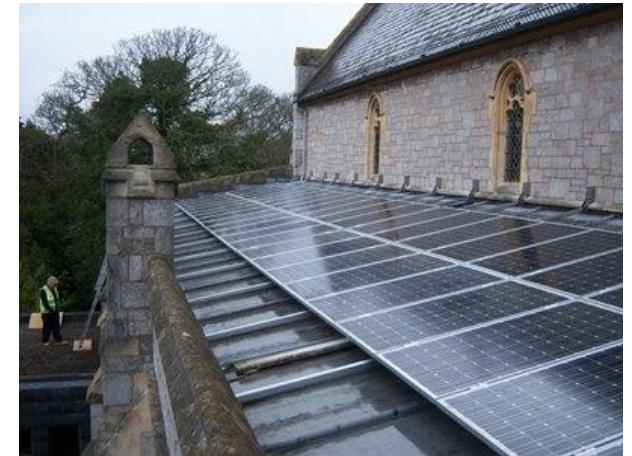
Photovoltaic panel array installed on south facing aisle roof
